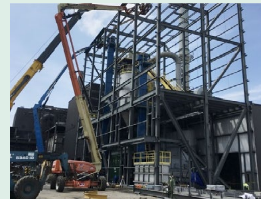
Sand recycling system.
