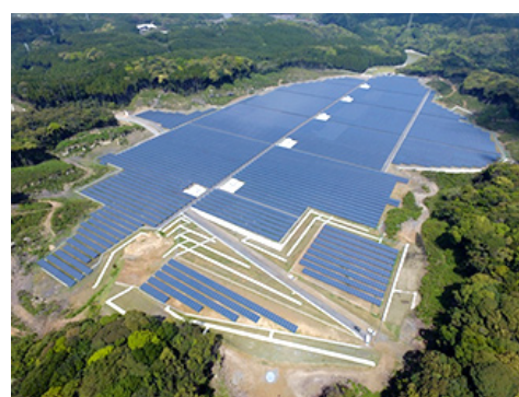
Saga-Ouchi Photovoltaic Power Plant
