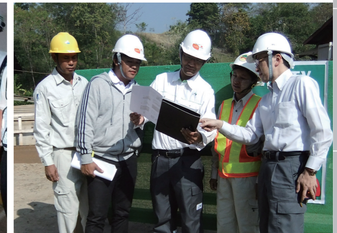
On-site supervision in project for capacity development of road bridge technology in Myanmar
