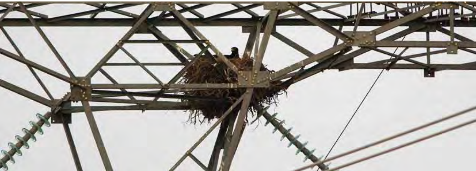
Black Eagle nesting on a transmission structure in the Karoo
