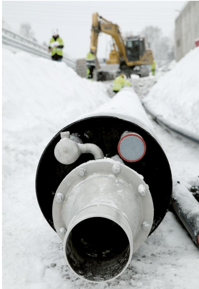
Locally-sourced and innovative heat generation: Heat is recovered at Myrvoll Station from sewage water in a specially designed pipe.
