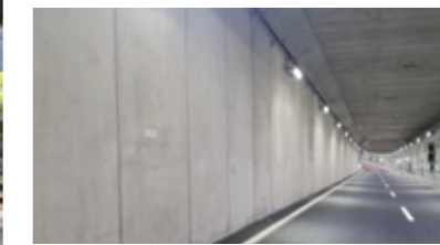
Labor/saving for construction of the "Large Section Box Culvert" by the "Hybrid Half Pre-casting Method": At the A-ramps for turn off of Keiyo Junction in Tokyo-Gaikan Expressway
