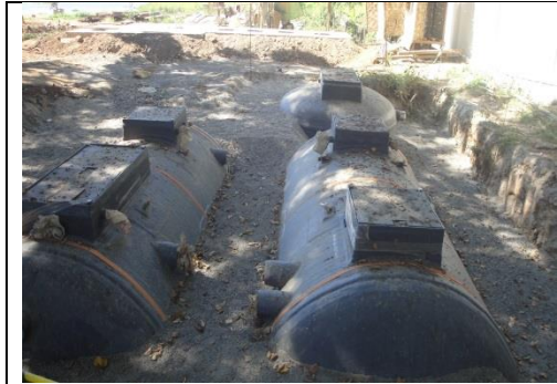
Wastewater treatment system
