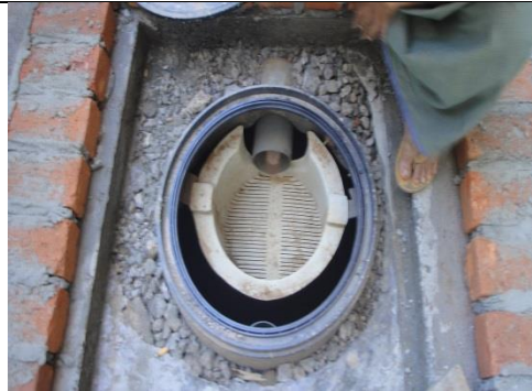
Grease trap system installed at Kitchen
