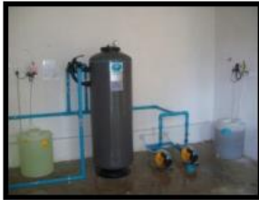
Sand Filtration & Chlorination
