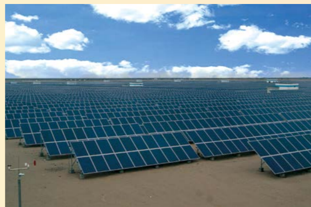
Datang Qinghai Golmud Photovoltaic Power Station, the first PV power project of CDT
