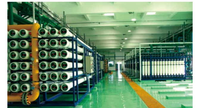
Seawater Desalination System of Wangtan Power Generation Company under CDT
