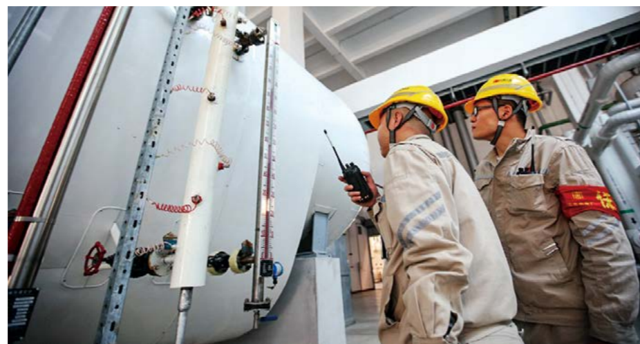
Beijing Gaojing Thermal Power Plant ensures safe and stable operation of the generating units during the "Two Sessions".
