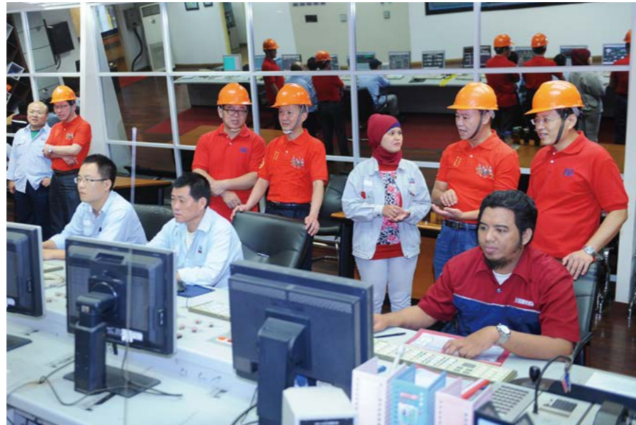
The Cilacap Power Station in Indonesia is the only energy base in southern Java. The operation, repair and maintenance of the base were entrusted to us.
