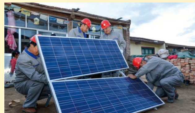
In Qinggenhe Village, Ziketan Town, Xinghai County, Qinghai Province, technicians of CDT are installing household power for users that had no access to electricity.
