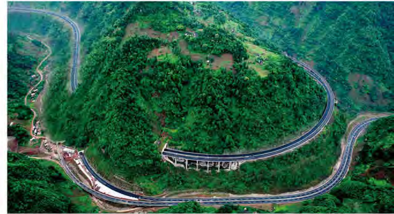
Shuifu - Malliwan Expressway Project financed by the Bank invented spiral extended line bridge and tunnel section.
