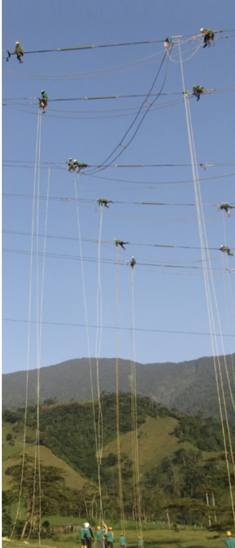
Maintenance of the Guavio-La Reforma line, in Medina, Cundinamarca. Our crew of linemen works at a height of 50 m following all occupational safety and health standards.
