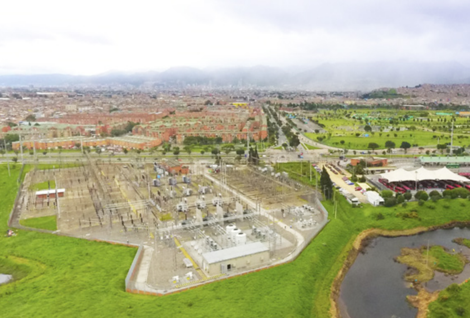
Tunal Substation, through which we supply energy to Bogotá
