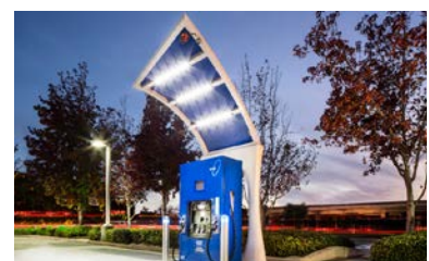
A hydrogen station operated by FEF
