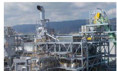
Konan Utility's wood biomass cogeneration facility
