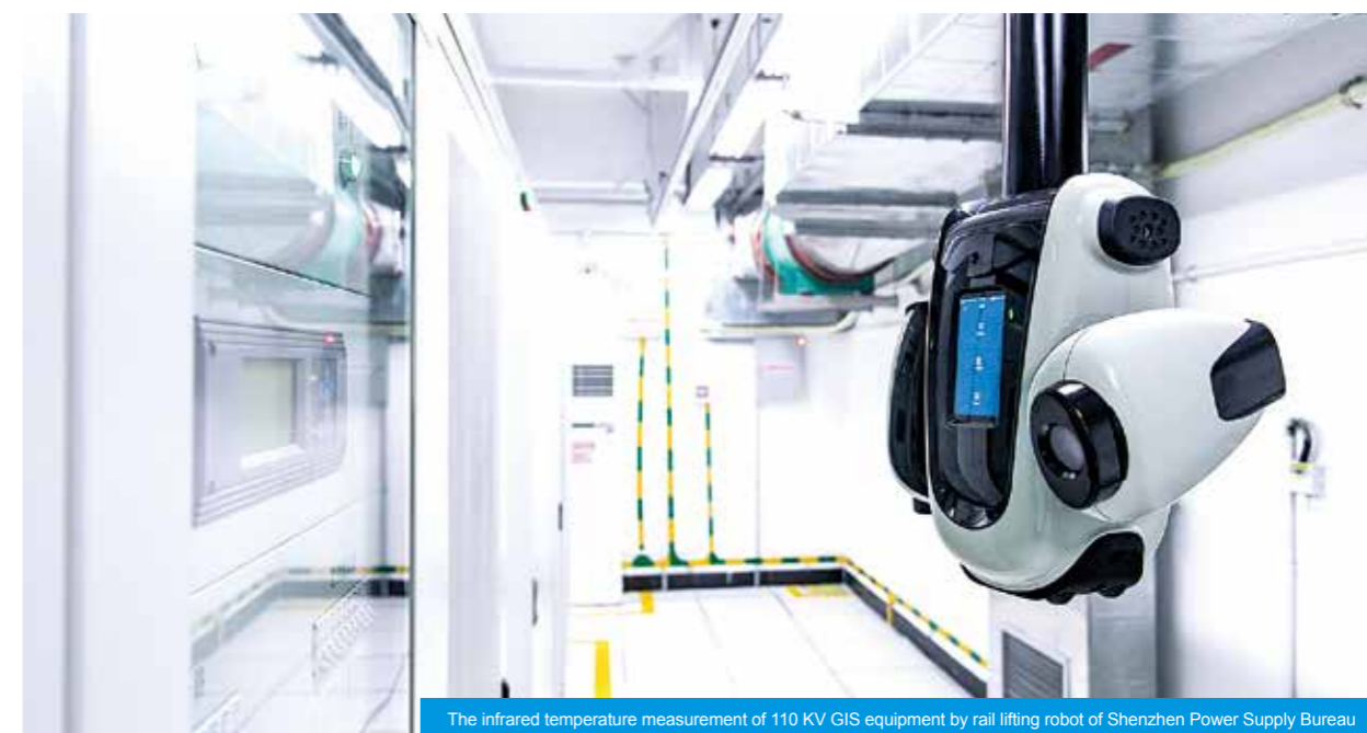
The infrared temperature measurement of 110 KV GIS equipment by rail lifting robot of Shenzhen Power Supply Bureau
