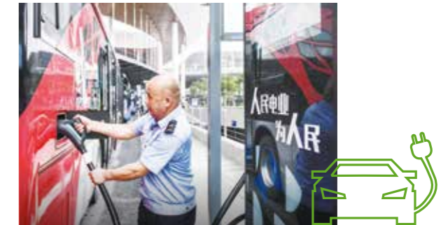
Charging piles for artificial island of Hong Kong-Zhuhai-Macao Bridge
