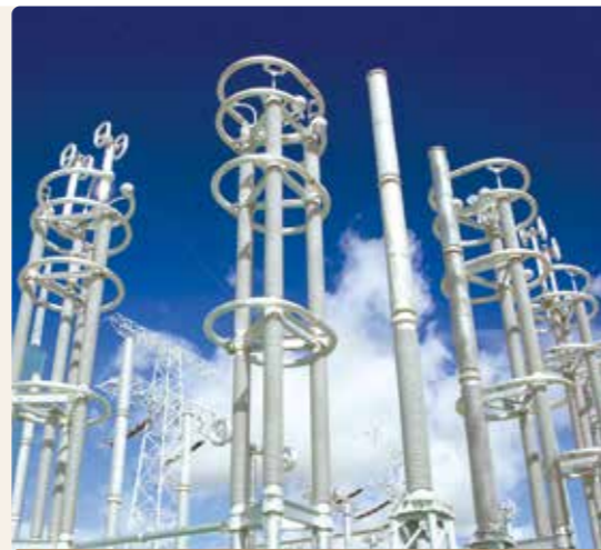
The sending end of ±800 kV Yunnan Northwest DC Project- Xinsong converter station, DC field
