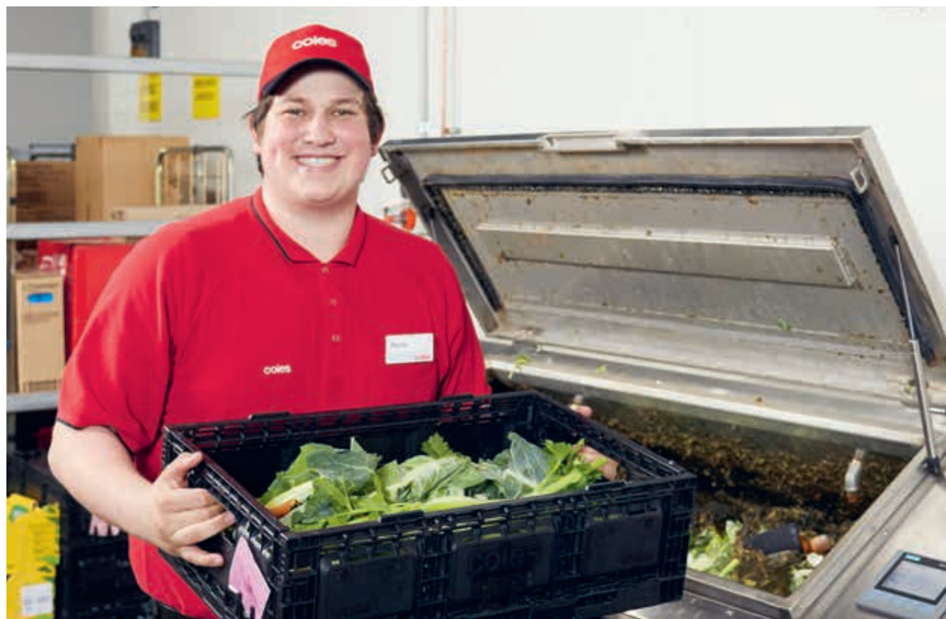
Coles Southland team member Xavier processes food waste with an ORCA food digester. The food waste is digested by the ORCA then sent to the local waste water treatment facility.
