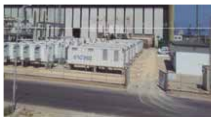
Litoral Almería Battery: Installation of Ion-Li Batteries at the Litoral de Almería Plant.
