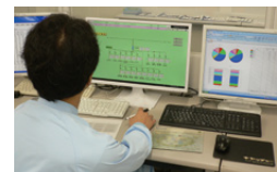
Power monitoring system of the Fukusaki Factory
