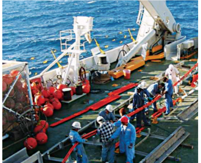
IPS Cable Systems Limited (Seacom)
