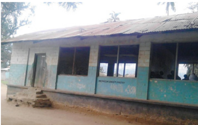
Mwembesongo primary school - renovations (before)
