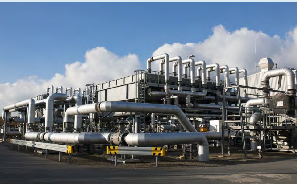
The Brammer compressor station is one of DEA's operational sites where we managed to achieve significant energy savings in 2018 by taking various technical measures.
