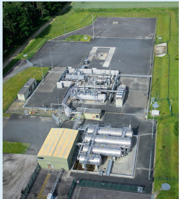
The 'Völkersen Z4' drilling site will be equipped with an ORC unit for the utilisation of waste heat.
