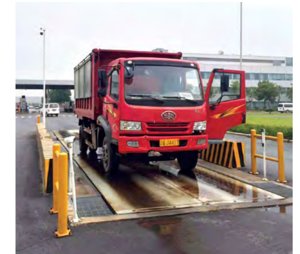
Newly installed waste weighing system.
