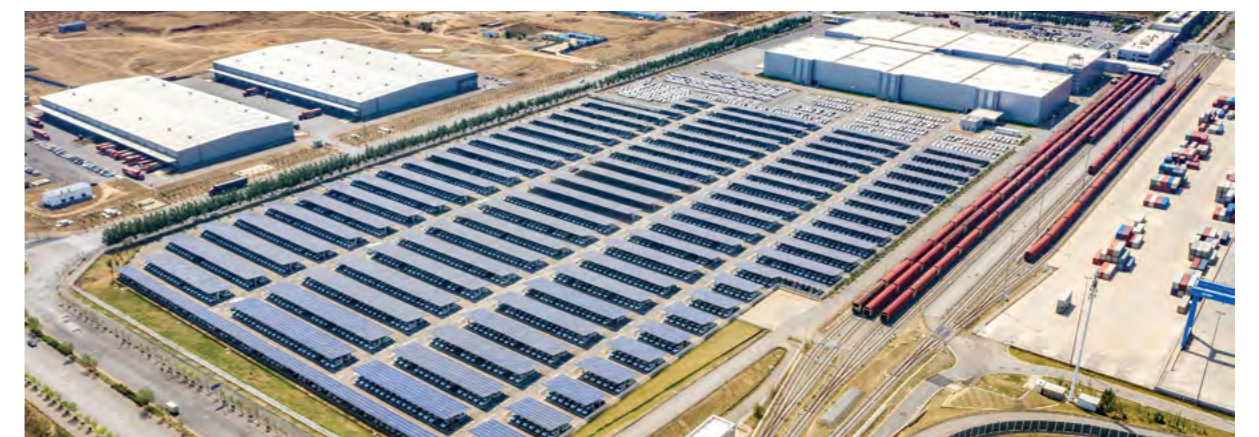
Solar panels at Tiexi plant.
