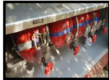
CO2 based Firefighting System
