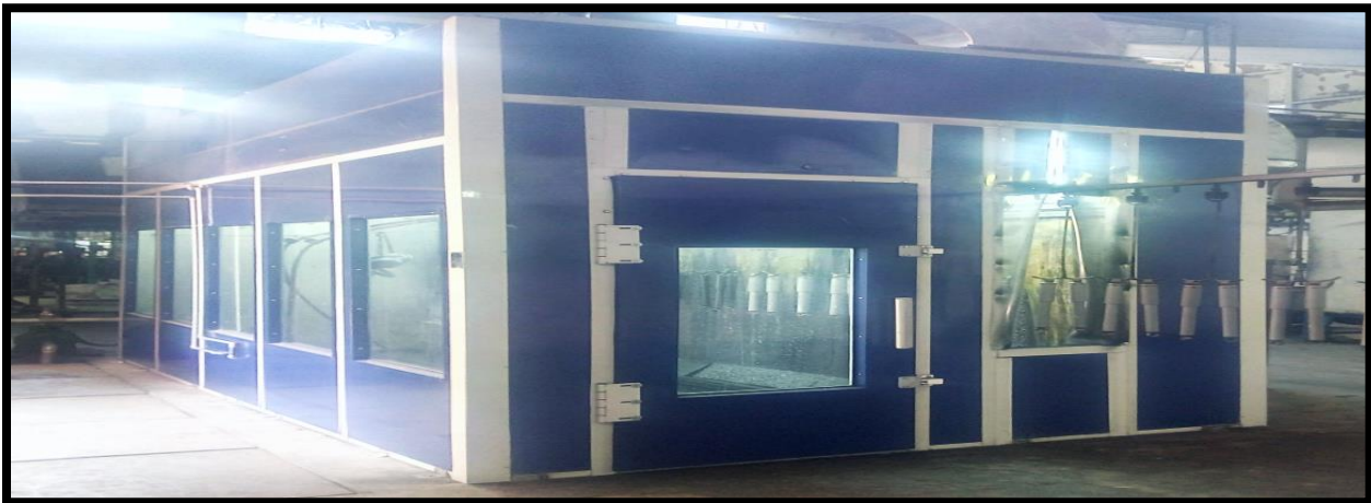
Newly Installed Paint Booth
