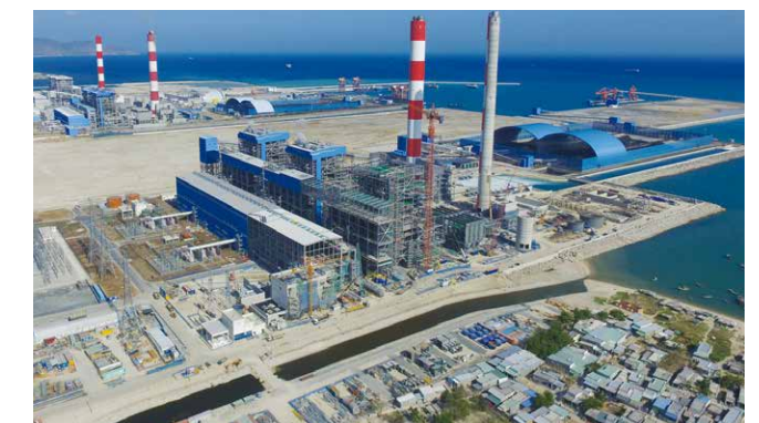
Vinh Tan 4 Coal-fired Thermal Power Plant in Vietnam
