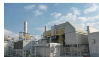
Gas-turbine cogeneration system introduced at the Sendai plant
