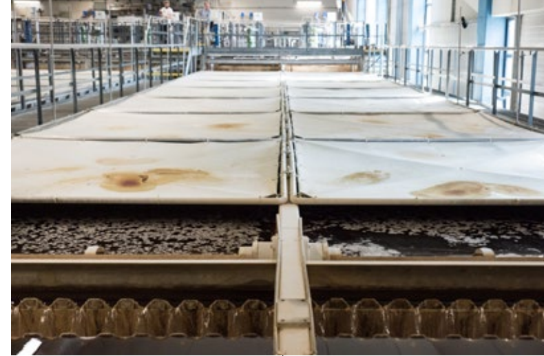
Waste water treatment facility, Wattens, Austria
