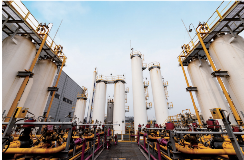
Hydrogen Gas Factory, Dangjin Integrated Steelworks
