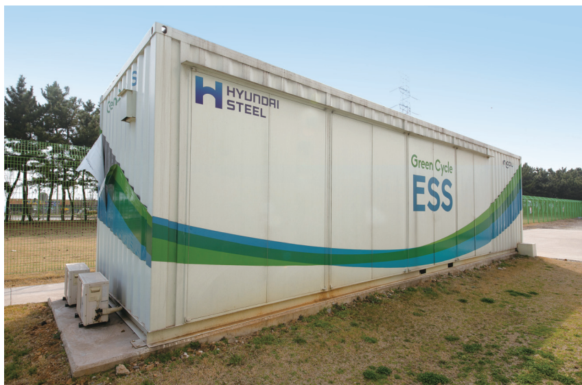
ESS facilities based on recycling EV waste batteries
