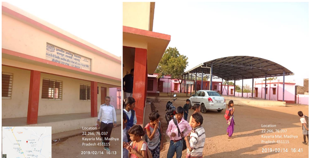
Figure 23 Construction of shed for mid-day meal and class room at Govt. School Charanpura
