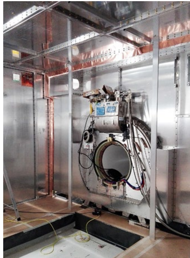
High-precision installation at customer site of one of Elekta Unity systems.
