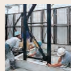
Creating safe, secure and comfortable housing together with the Sekisui House Association
