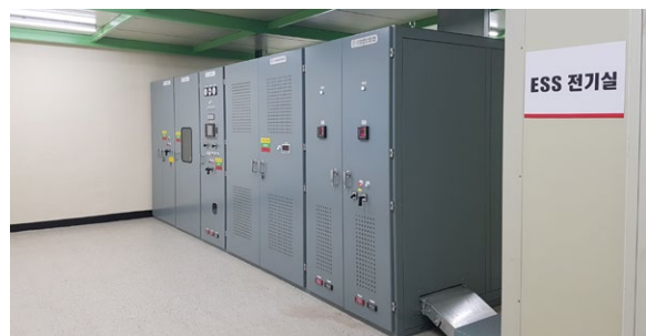
ESS (1MWh) for Emergency Generator Replacement at POSCO ICT Pohang Works
