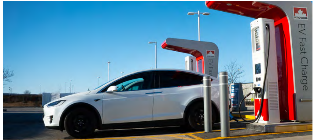
Petro-Canada electric vehicle charging station in Milton, Ontario.
