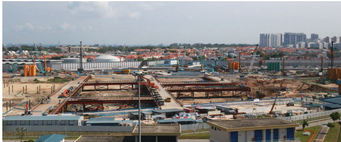
▲ T301 worksite in Singapore where GS E&C has been working with partners
