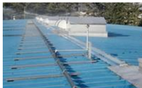
Running status of circulating roof spray system
