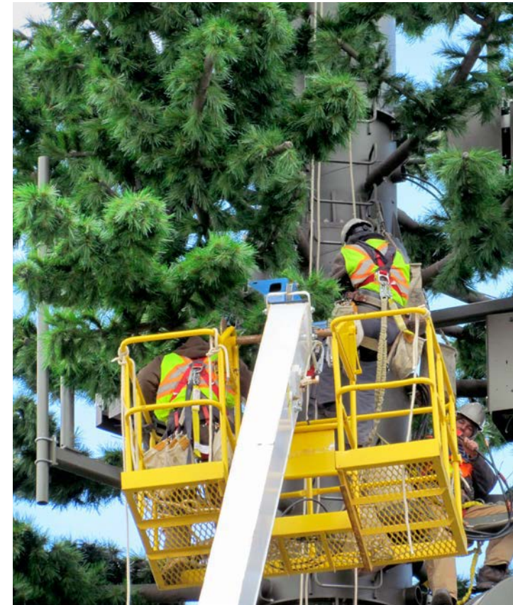
First and Only Canadian designed pine tree in Milford Bay (Muskoka), Ontario. One week was required to complete the build. In this picture the rigging crews are making the final connections between the radios and the antennas.
