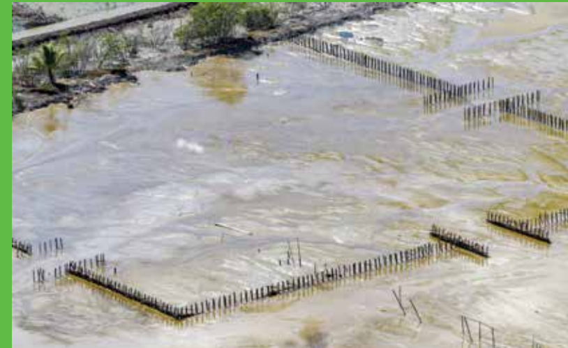
Sediment Trapping Units installed along the coast of Suriname promote sediment deposition and create conditions for halting and reversing erosion, including by creating a habitat for new mangrove juveniles.
