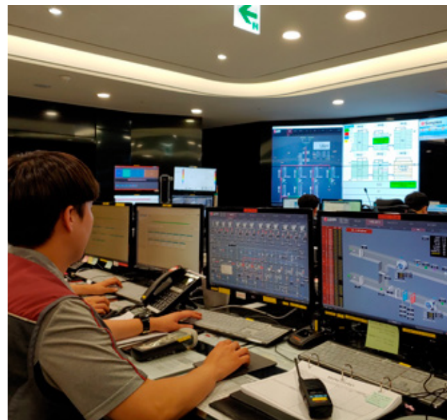
LG Science Park Control Center equipped with a solution for integrated building controls and energy management
