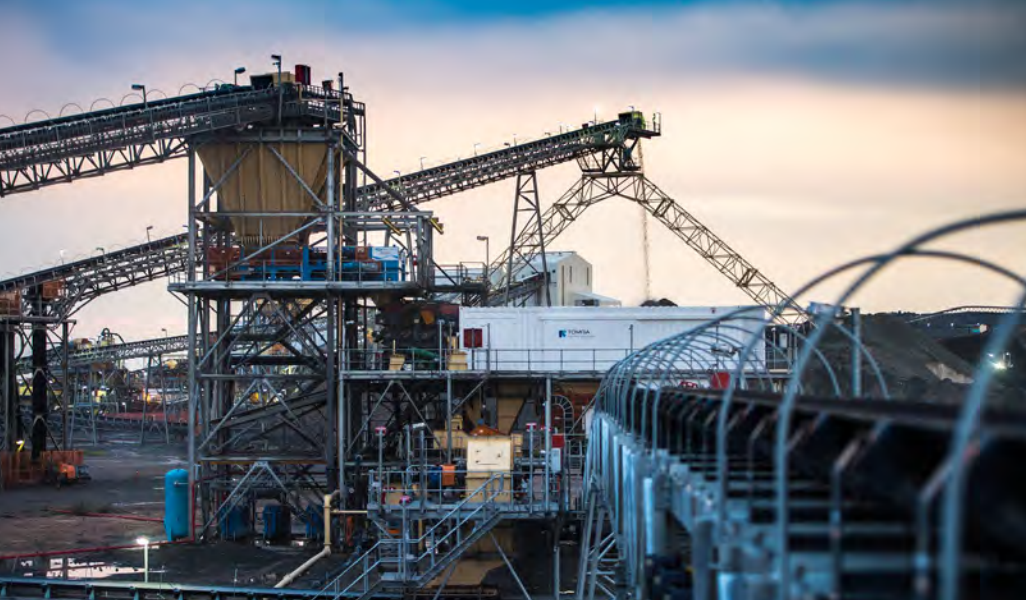
Mega Diamond XRT (X-ray transmission) facility or MDR (mega diamond recovery) unit
