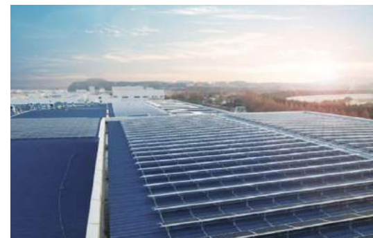
Photovoltaic power generation facilities at the Namyang Technology Research Center
