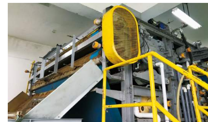
Sludge dehydrators at the Ulsan Plant
