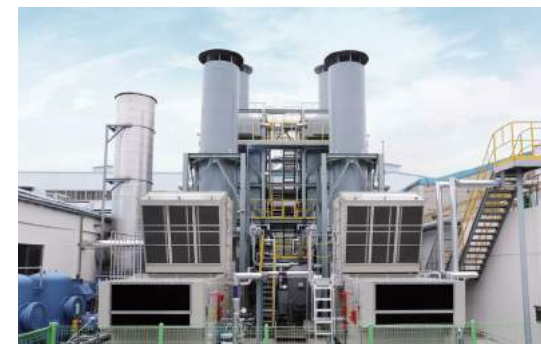
Co-generation facility at the Ulsan Plant
