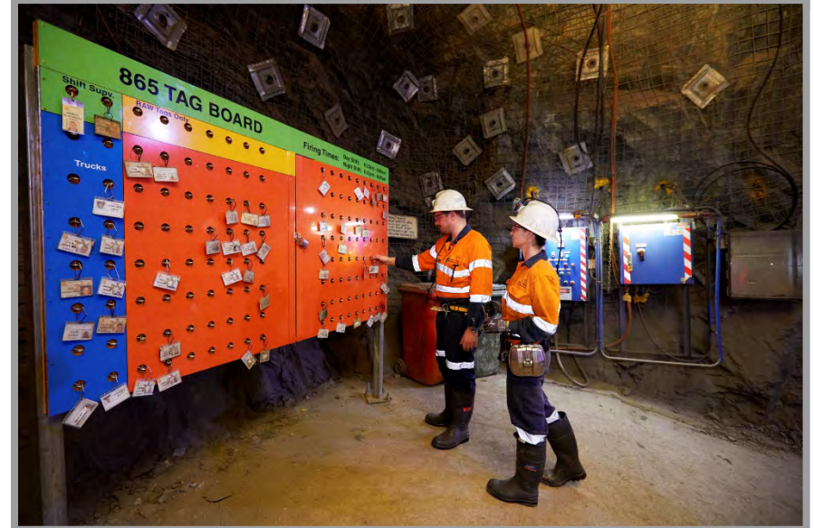
Above – isolation tag in an MCC room at Gwalia, WA.
