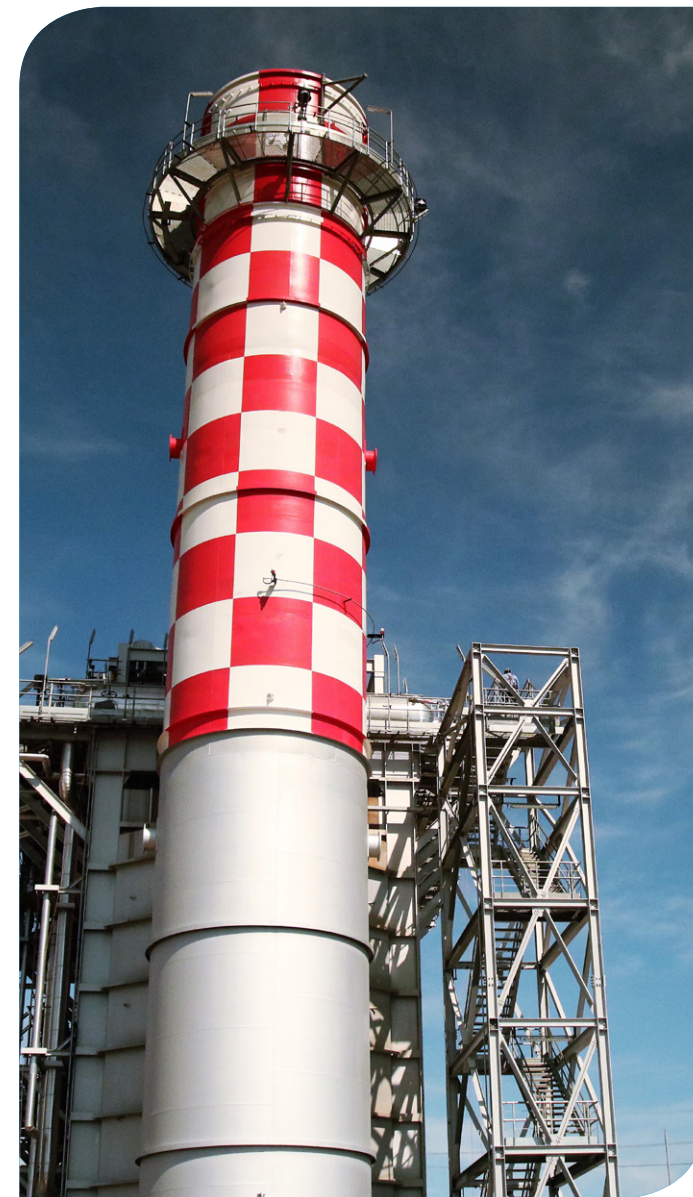
TPP Mauá 3. Eletrobras Amazonas GT / Alessandro Nunes collection
