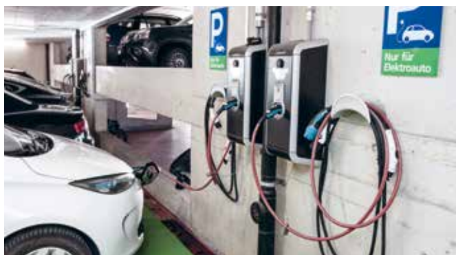
Clients and employees can charge their electric cars in the parking garages at various locations.
