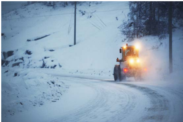
The roads on the Romaine-4 jobsite are maintained by a company from the region, under a contract awarded by Hydro-Québec.
