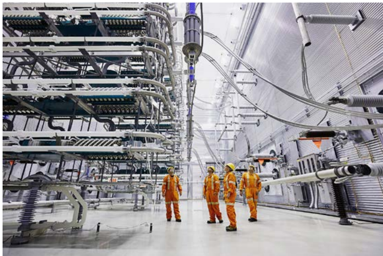
Outaouais substation, the main component in the 1,250-MW interconnection with Ontario. Hydropower exports avoid the emission of substantial quantities of GHGs.
