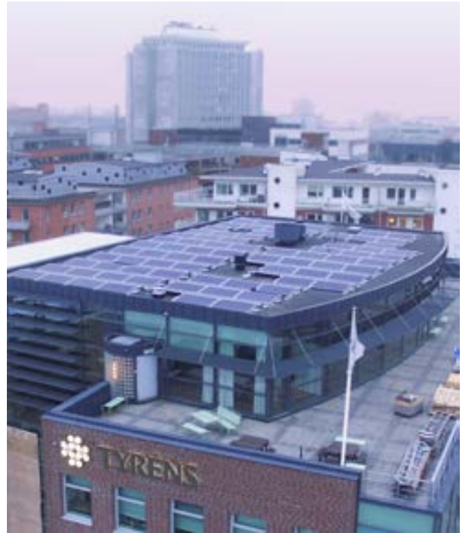
In conjunction with the redevelopment and extension of Tyréns premises in Malmö, we installed 154 solar panels on the roof.
