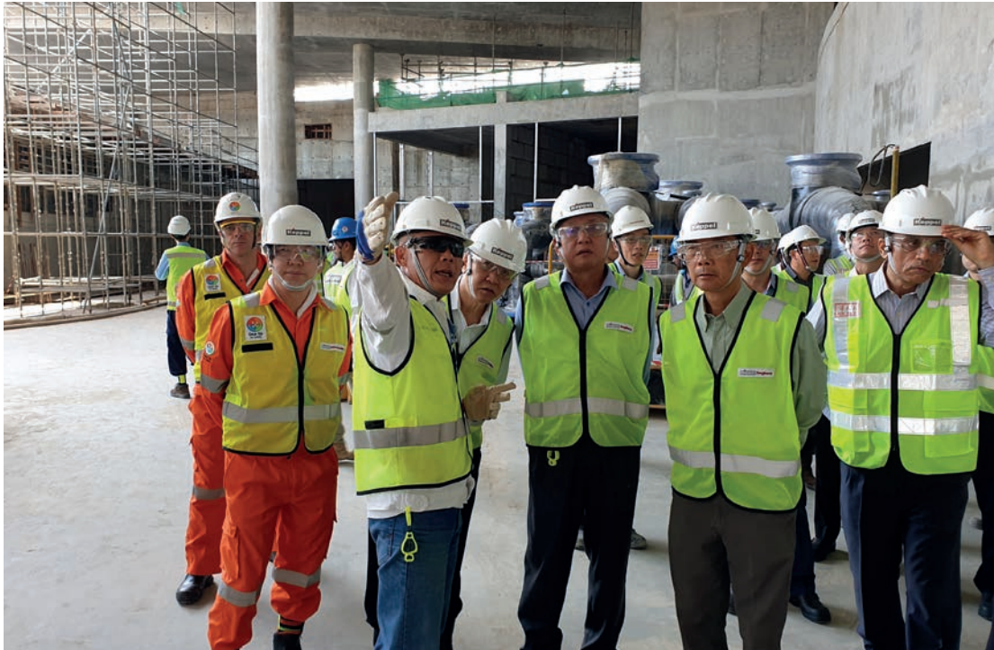
Keppel's Board Safety Committee regularly makes site visits to the Group's operations such as the Keppel Marina East Desalination Plant in Singapore.
