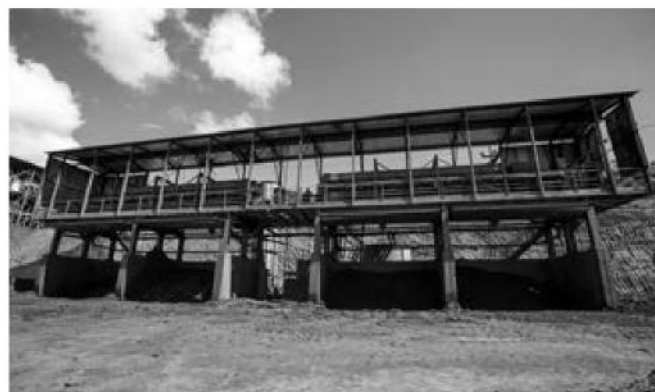
Installation of press filters
