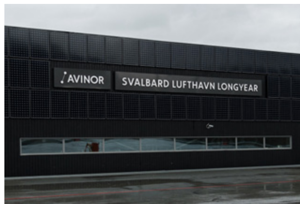
Solar panel array at Svalbard Airport.
