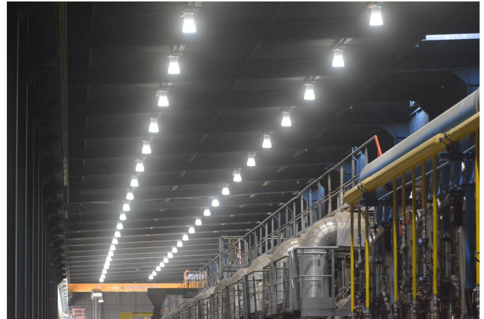
The new LED-enlightened halls in Genk.
