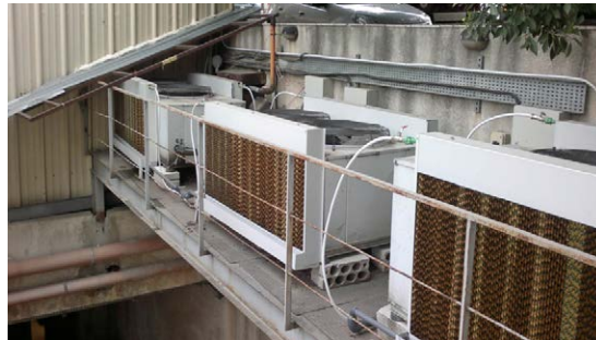
Implemented Evaporative Cooling.
