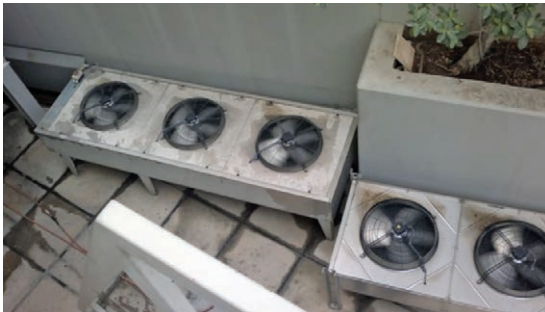
Condenser units in Fassouh Headquarters.
