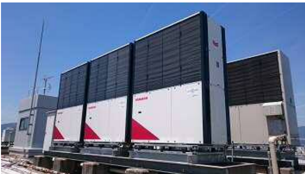
Upgraded air conditioning unit (outdoor unit)
