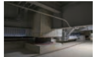
Seismic isolation equipment of the Disaster-Resistant and Eco-Friendly Warehouse (Seishin Distribution Center, Kobe)
