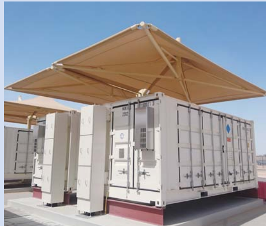
NAS batteries installed in Dubai
