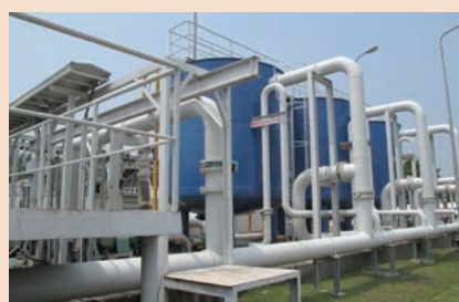
Facilities for a plant wastewater zero system
