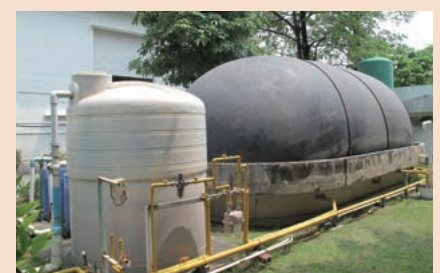
A storage tank for biogas
